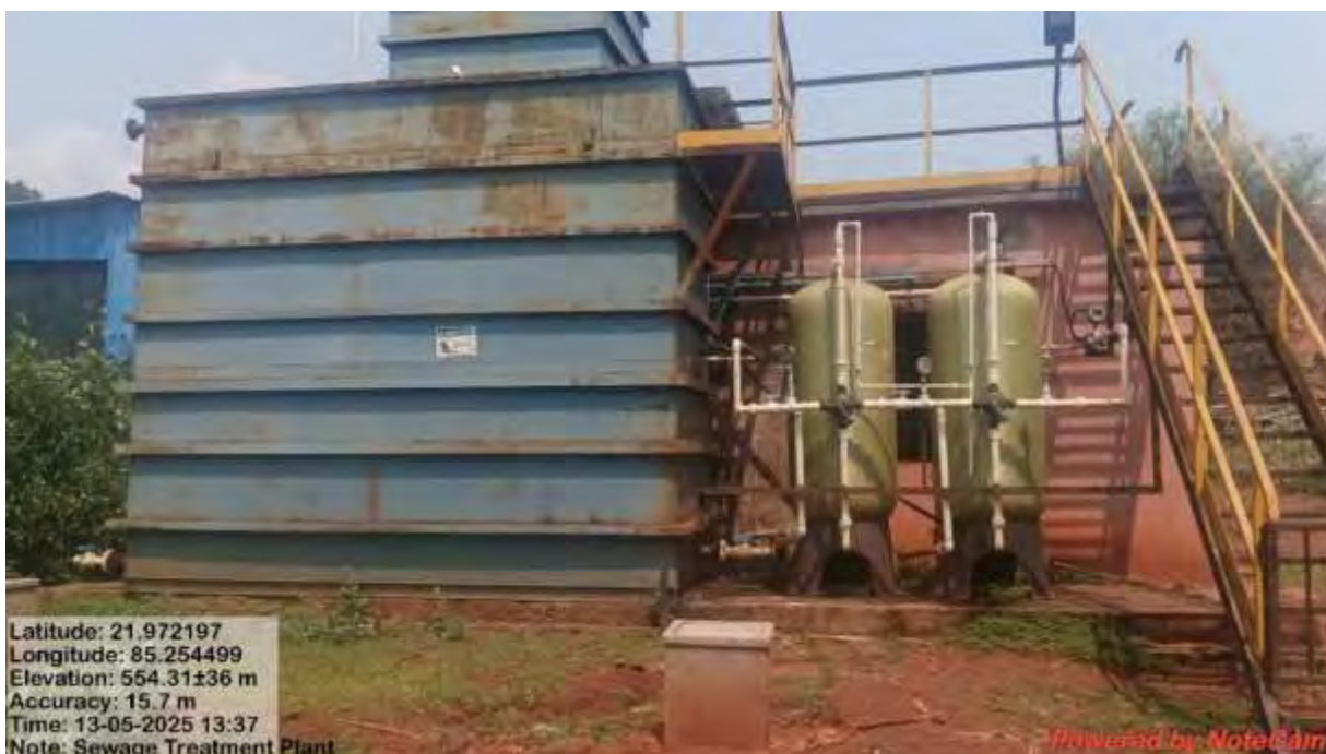
Figure - 26: 60 KLD STP in Nadidihi Iron and Manganese mines
